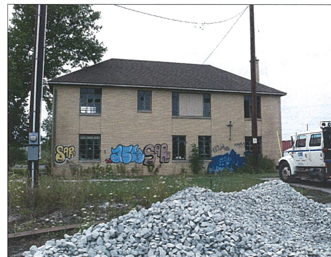
East side graffiti. Note new roof, thanks to Pete Frantz!
