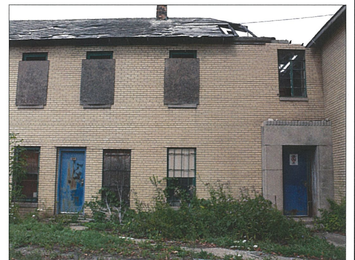
Annex roof damage above office entrance.
