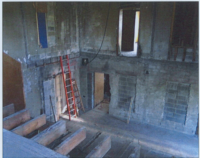
Half of the second floor has been removed. Now we'll build brand new framing to replace the old portion. Note old window placements blocked in with the 1950 era addition.
