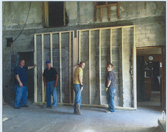
After framing in the east wall of the original building, they'll frame two more walls, insulate them, and move on to building the frames to support the new second floor.
