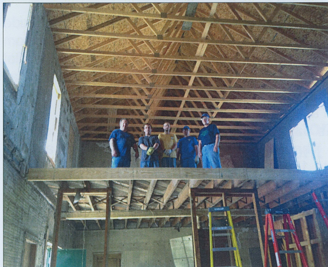
The Ripping Crew (L2R): Jack, John, Bill, Chuck & Bruce. They've just nailed a 2x12 face board to the one half of the undamaged second floor.
