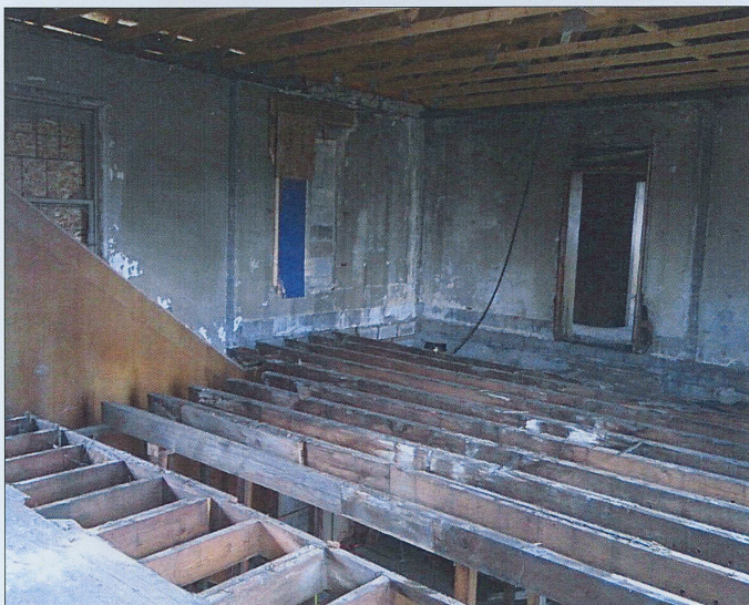
The water-damaged rafters are exposed and half of second floor sheeting has been removed. That door leads to the board room. That wall with a sloped veneer lines the stairs.
