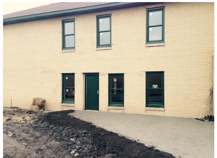
No more tube steaks gang; it's "Shrimp on the Barbie!" Check out the new soffits up top matching our new windows!
