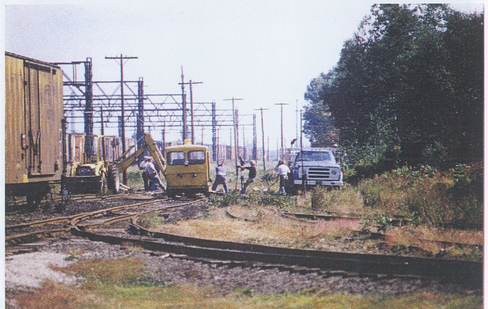
He's leaning on that lining bar as another man drives a spike home. In the 1980s, a small backhoe made the work easier.
