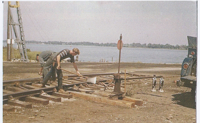
Two Simplex jacks stand next to the blue Dodge Powerwagon near the high mount switch stand.
