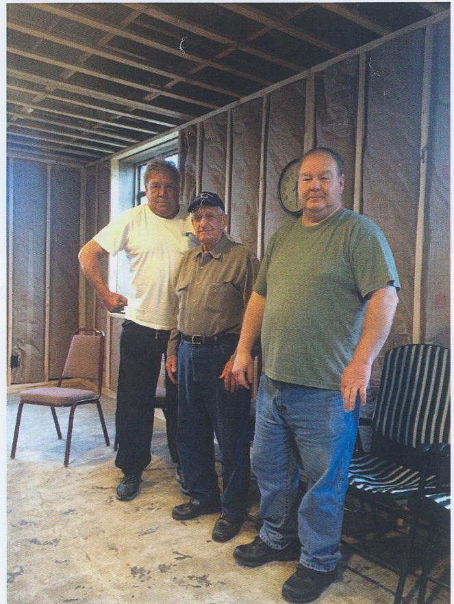
The heavy lifters: (L2R) Dave Schultz , Bruce Sawdon , and Jack Allison helping to renovate the Agent’s office.
