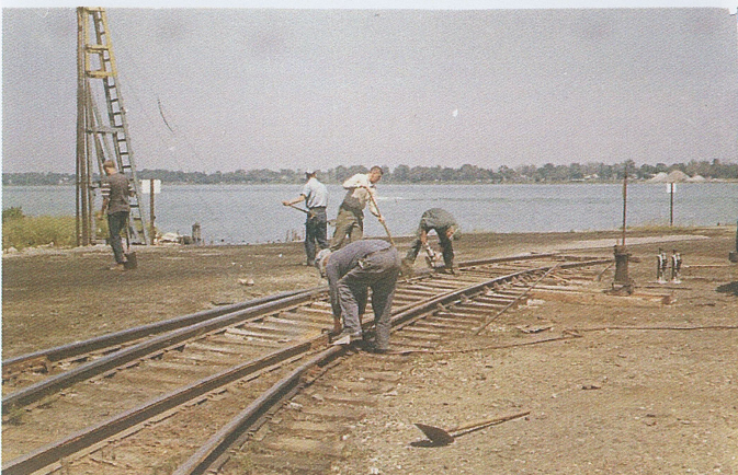
The gang has just replaced a switch point which is being ground with a grinder as more loose gravel is brought in.
