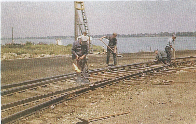
A torch is brought in to heat up angle bar bolts as the men try to feed loose gravel into that Diamond Crystal switch.
