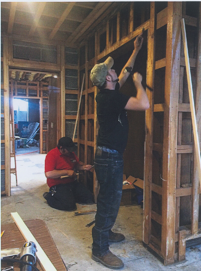
Society volunteers Andrew Armstead (L) and Bill Rauli chisel away excess glue to reach an even plane for drywall.
