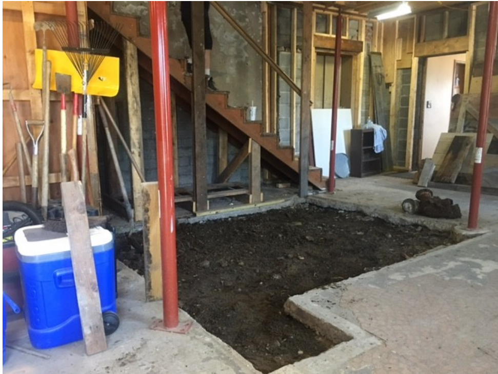
With a new cement floor, we'll be able to install a new wall with a double door leading into a future gift shop counter.
