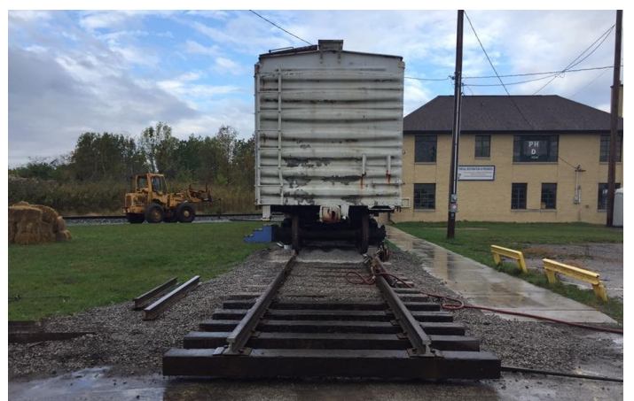
The track has been extended to the east right up to the edge of the parking lot. All that remains is more ballast.
