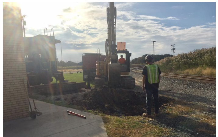
Pat Mike brings in several loads of ballast before the crew lays the ties.
