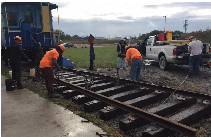
The crew from Armond Castle are preparing to spike each tie plate on the western extension of the display track.
