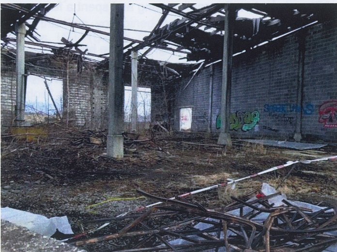
This is the three-bay Maintenance of Way portion used by the section gang. It's now the only structure left standing. (Photo: William Rauli)
