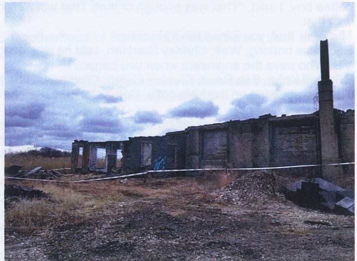
What's left of the 98 year old roundhouse: the north wall. Fortunately it contains the different patterns of brick and block that can help date & rebuild. (Photo: William Rauli)
