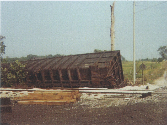
This was taken a few days later at the crossing. Note the fresh ballast and the brand new ties.
