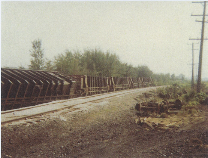
Hulcher has removed the hoppers and their wheelsets to allow the section to restore service. Note fresh ballast.
